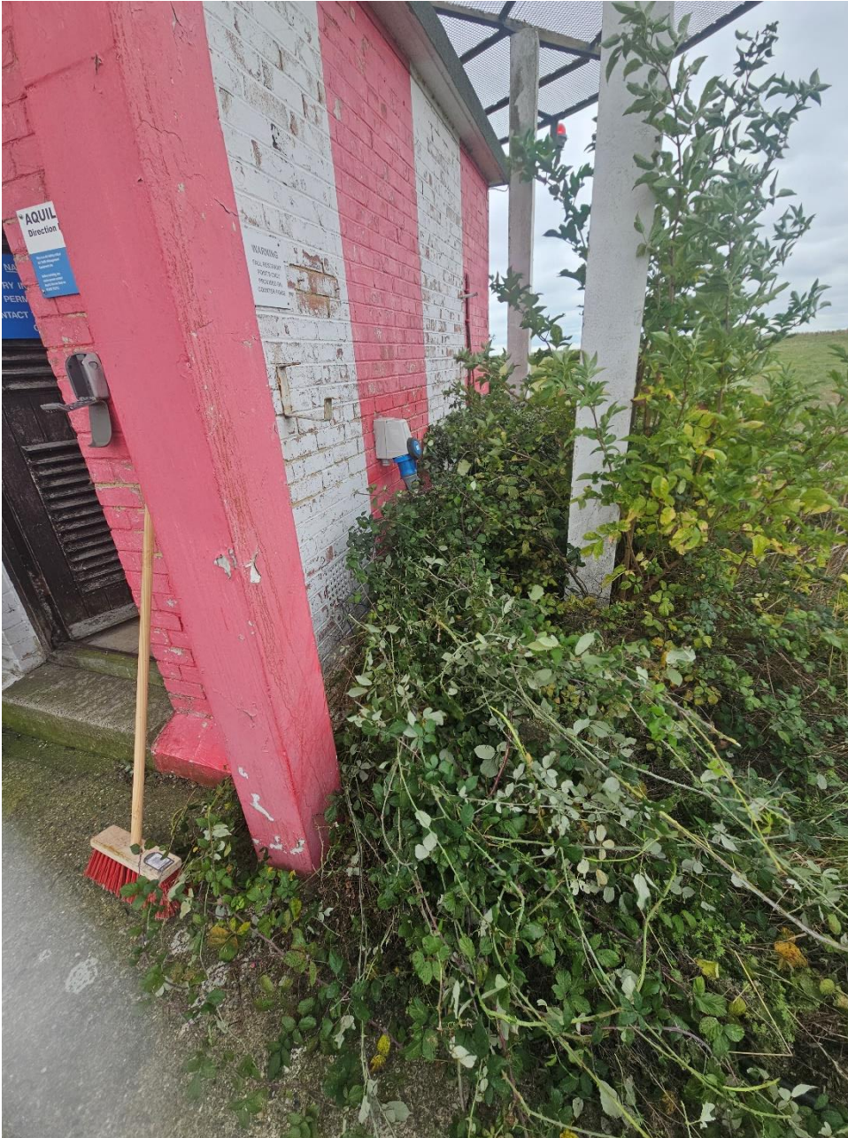
Image A – Overgrown Vegetation
